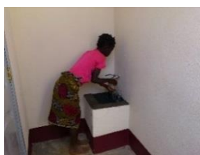
Water tap placed inside privacy wall
